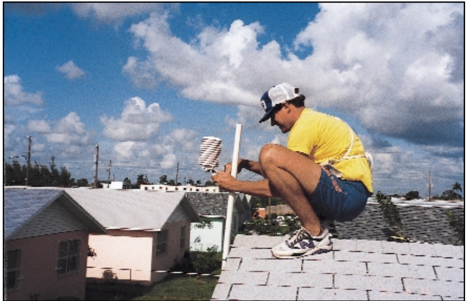
FSEC assistant John Broughton installs sensors on the roof of one of the monitored homes.
