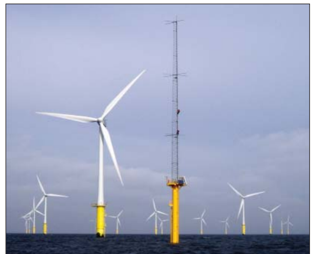
A Campbell Scientific datalogging system monitors this offshore wind farm located between Rhyl and Prestatyn in North Wales at about 7 to 8 km out to sea.
