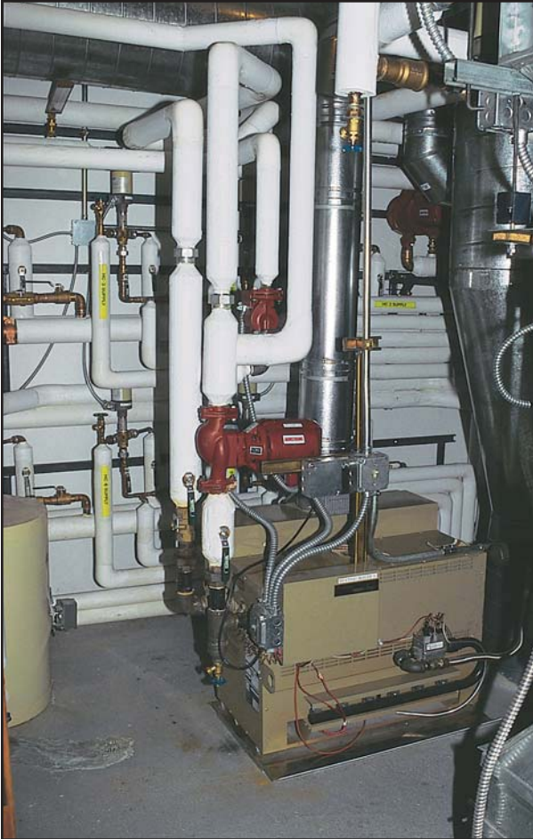
The CR23X monitors and controls the pumps, fans, and starter motors in an HVAC system.
