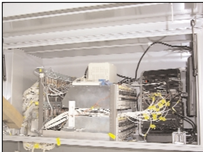
(Top) An enclosure housing a CR9000 system is bolted to a floor beam underneath the Williamsburg Bridge in New York City.
