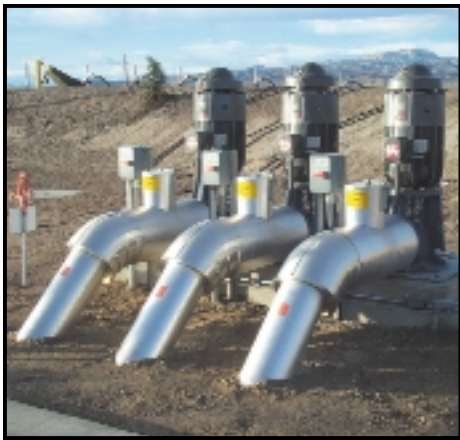
The operation of irrigation pumps is controlled by a datalogger digital I/O ports while flags trigger alarm call-outs to cellphones. Water Reuse Facility, Silver Springs, NV, USA
